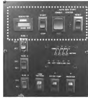
Command Center Panel
