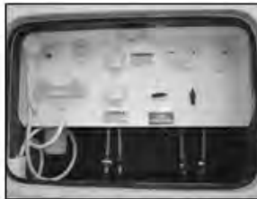
Fig. B Utility Center
